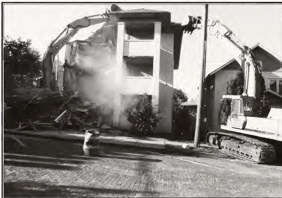
Onlookers were either elated or teary-eyed as the almost-human back hoes tore into Tiger Hall. The decaying dormitory was destroyed to make room for additional parking.
